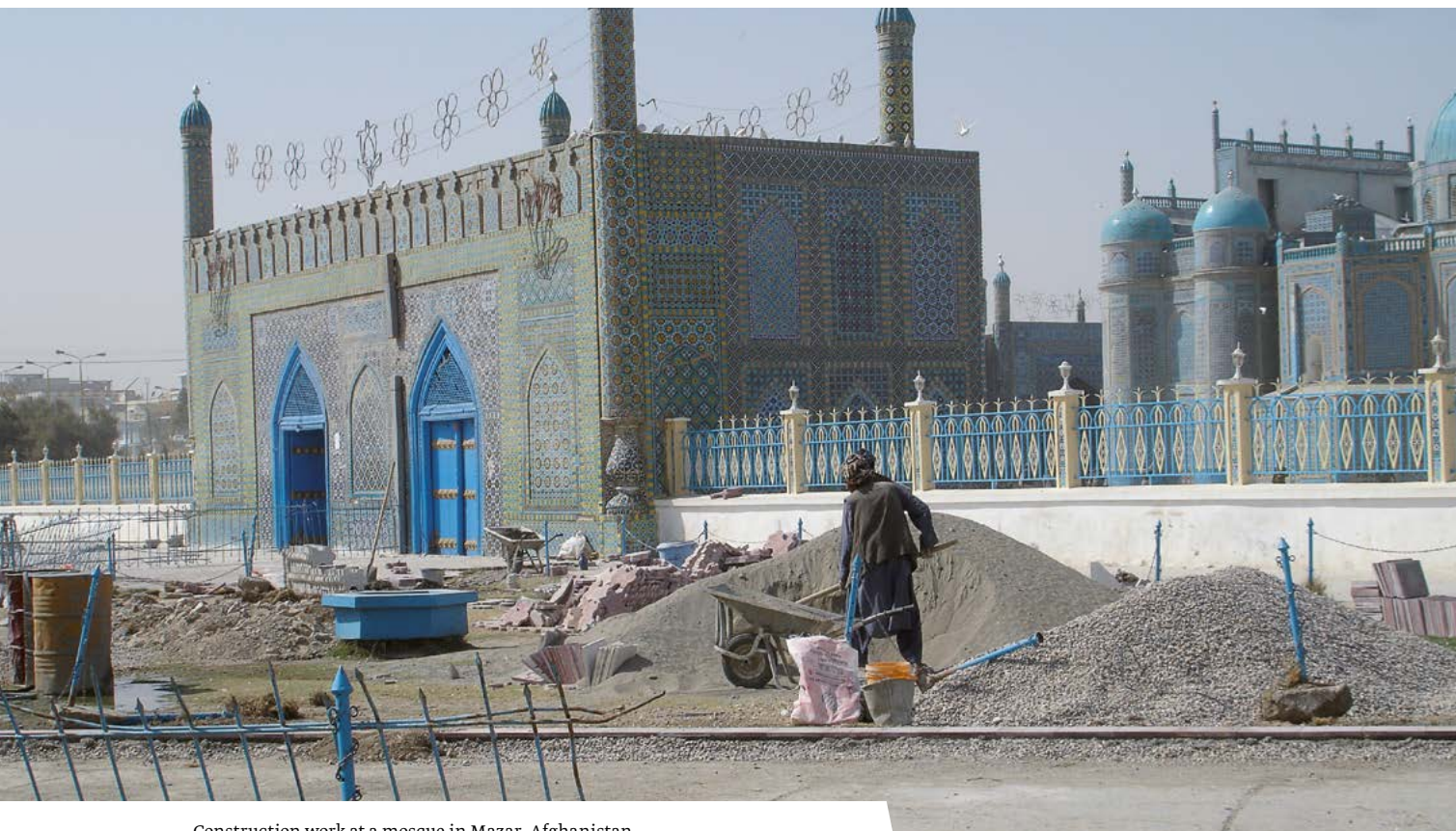
Construction work at a mosque in Mazar, Afghanistan Bauarbeiten an einer Moschee in Mazar, Afghanistan
